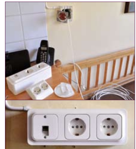
Figure 2: The upper photo is from the installation phase with POF on the floor. The old and the new power outlets are seen on the table. The lower photo shows the final result – the POF is hidden for the tenant, but broadband is available at each power outlet in the apartment.
